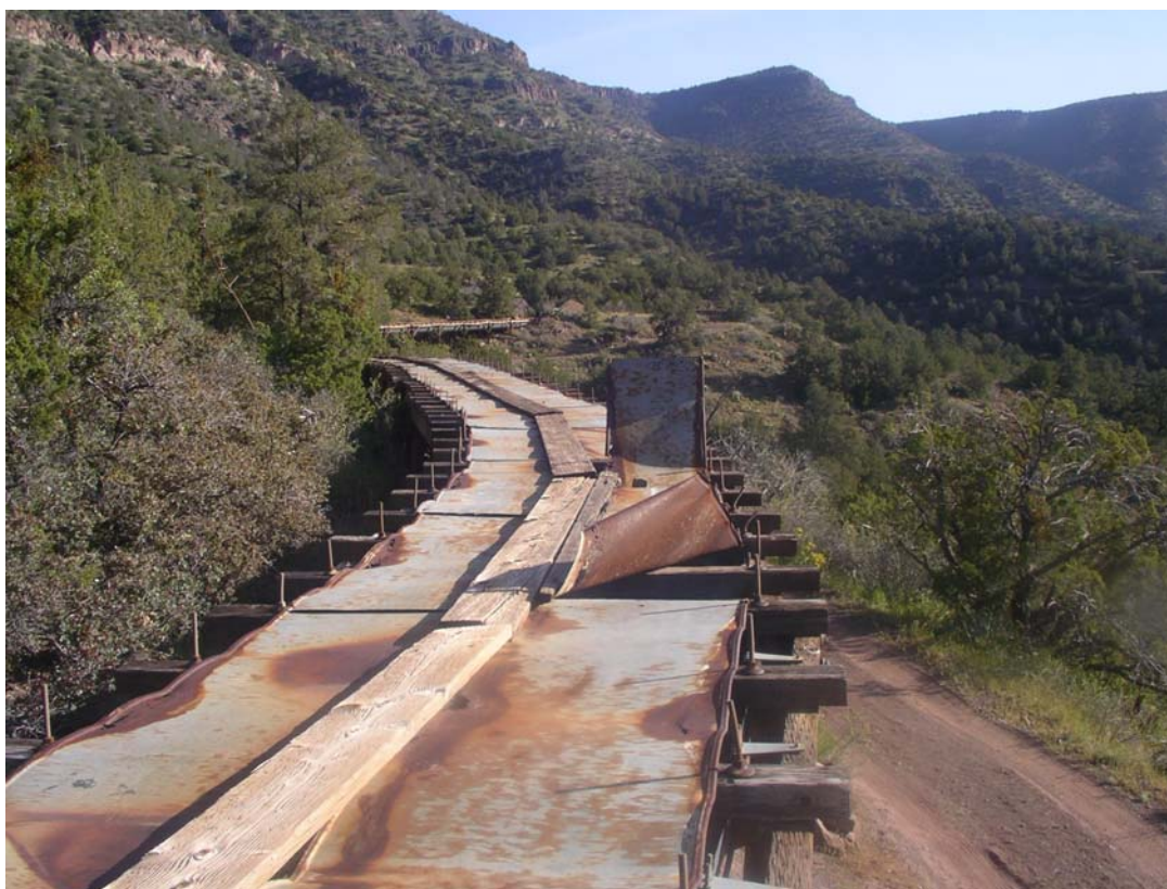
Photo 3. Flume that carries water from Fossil Creek to Irving Power Plant (looking up canyon; 14 April 05).
